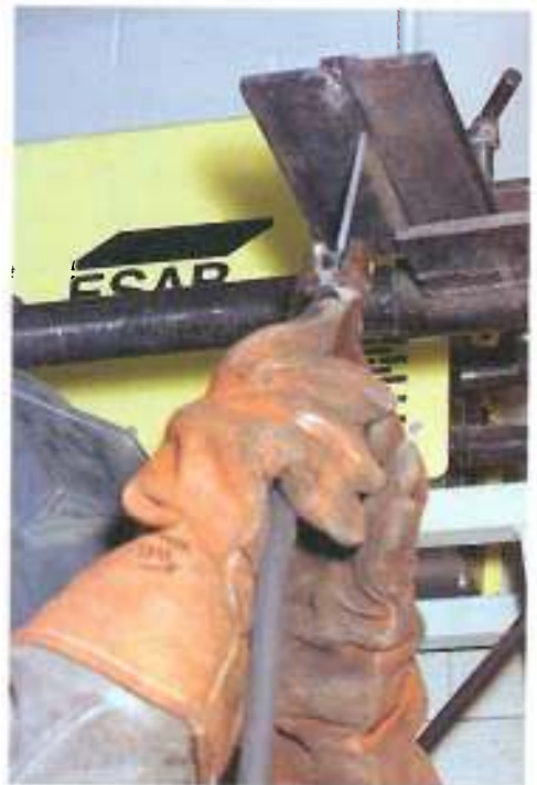
Figure 15-4. A welder may use both hands to hold the electrode when welding in overhead position.
