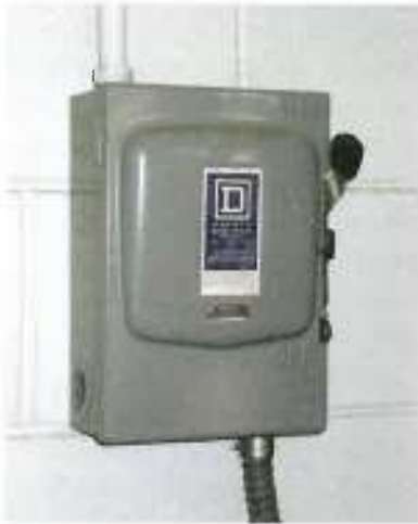
LOCATE POWER DISCONNECT NEAR WELDING MACHINE
