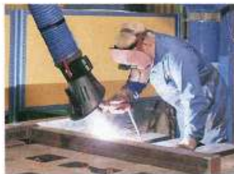
Figure 2-3. A ventilation system is required to remove toxic fumes, smoke, and dust caused by welding.
