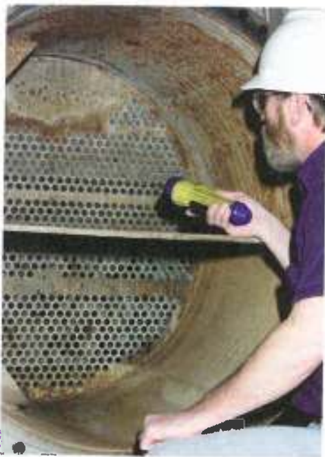
Figure 45-12. Repairs made to a heat exchanger tube-to-tubesheet joint are classified as pressure vessel repairs because they involve welding directly on a pressure boundary of the heat exchanger.
