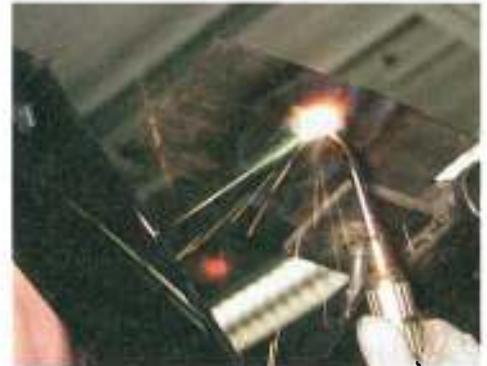
Figure 7-2. The filler metal moves ahead of the torch and distributes the molten weld pool as it is moved.
