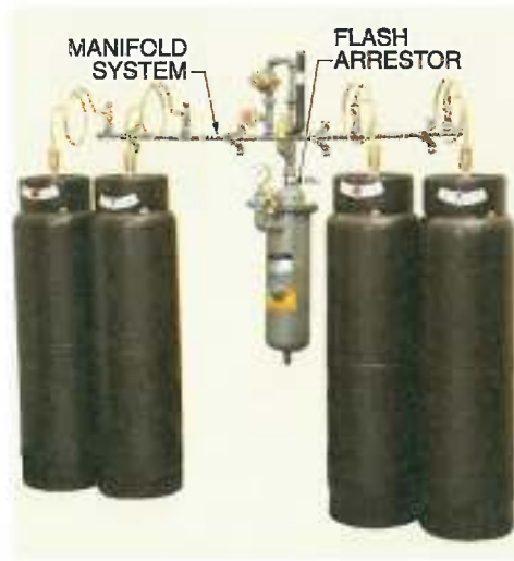
Figure 4-4. Acetylene cylinders are connected to a manifold system in areas where a high volume of welding is to be performed.
